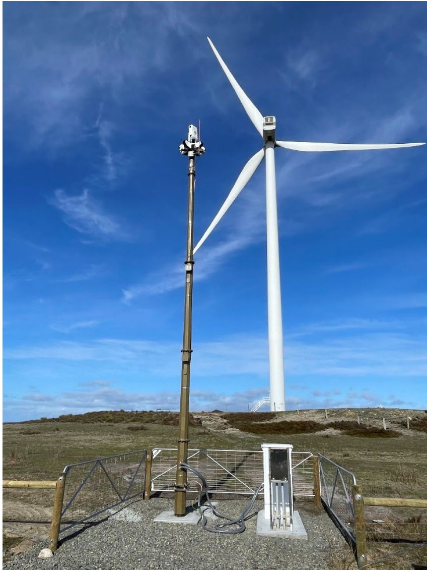
Figure 5. IdentiFlight system installed at Musselroe Wind Farm
